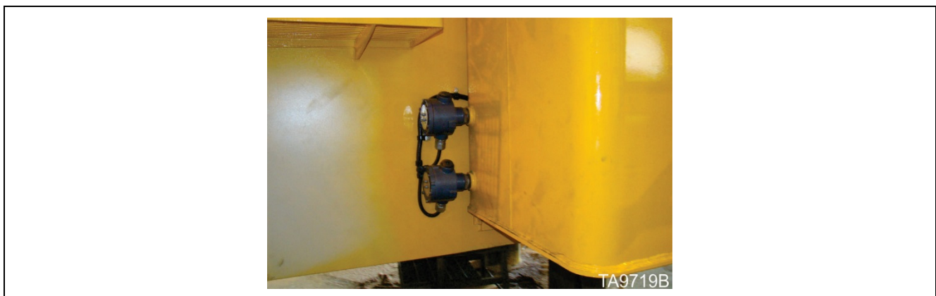
Figure 3. Hydraulic reservoir heaters (typical)
